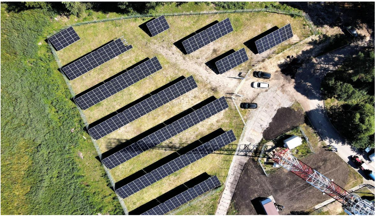
Photovoltaic installation for the Municipal Sewage Treatment Plant and education facilities, source: Kalety City
